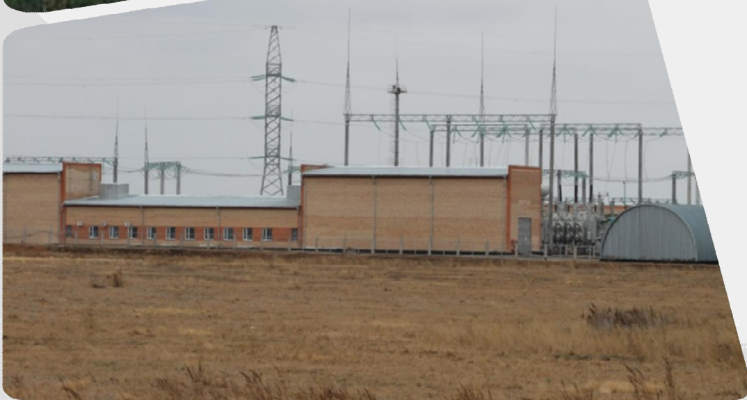
SUBSTATION 220/110/10 KV "DOSTYK"
