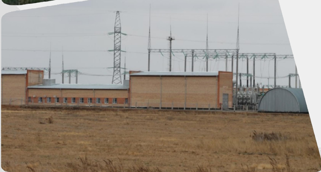
SUBSTATION 220/110/10 KV "DOSTYK"
